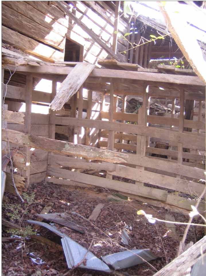
Photo 18. Barn, interior south side, view east. This area appears to have functioned as animal pens. Planks have been laid over the central pen, which is accessible from the doorway in the log section at left.
