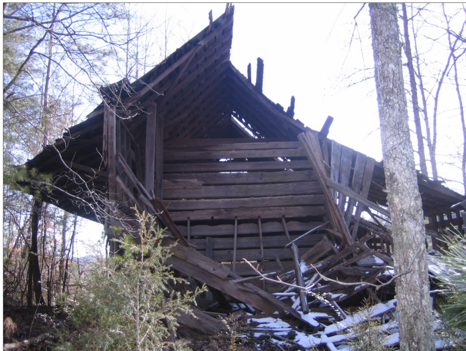
Photo 15. Barn, view east. Because much of the western frame extension has collapsed, the core log structure is visible.
