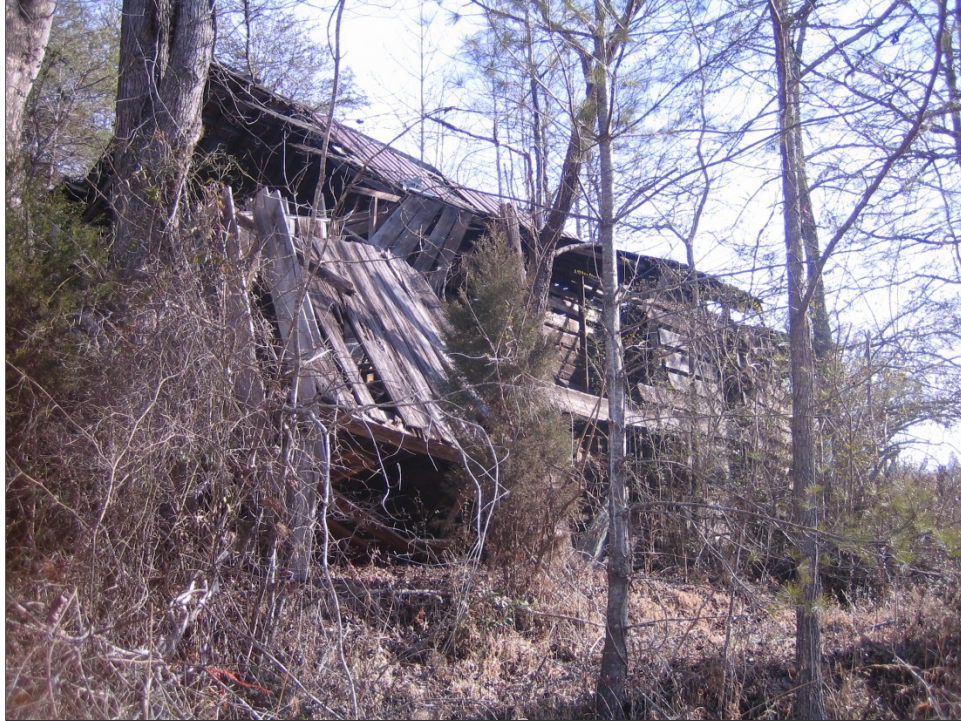
Photo 16. Barn, south elevation view northeast. The left floor of the collapsed west end is visible at left.
