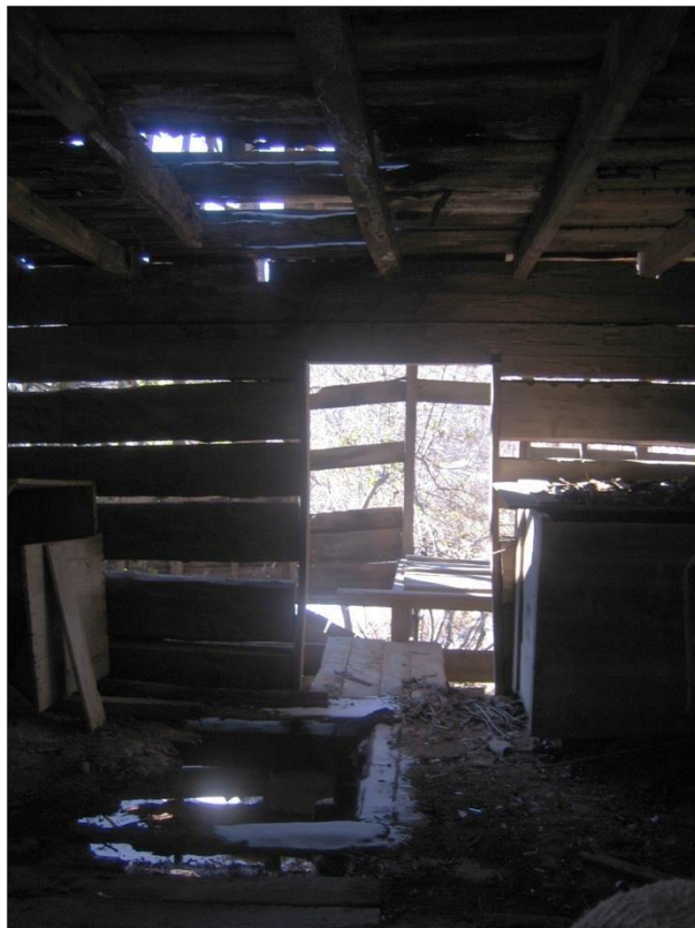
Photo 17. Barn, interior, view south. This view through the log building from the north entry shows deteriorated flooring at each level, and the south doorway to plank covering over a stall in the frame addition.
