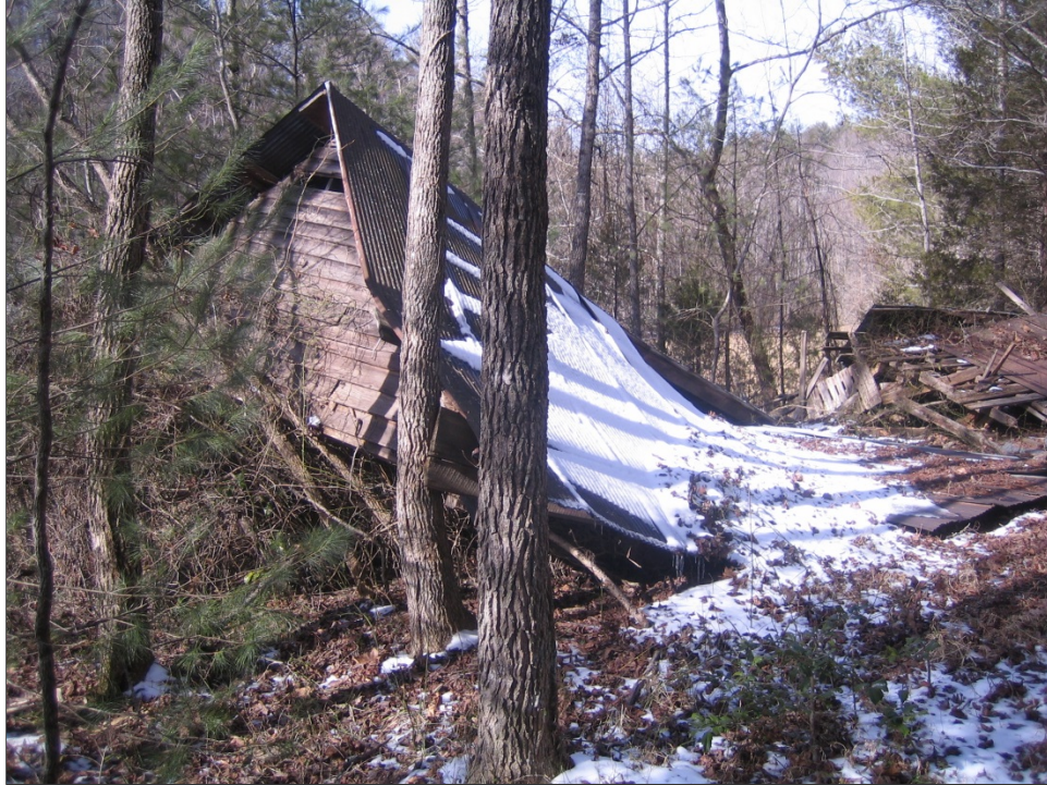
Photo 19. Former latched crib, now collapsed, view southwest.
