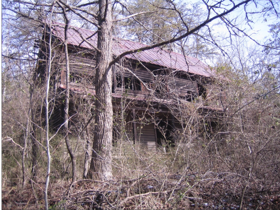
Photo 4. House, view northeast. Note the missing weatherboard at the second story, and missing door and window muntins.
